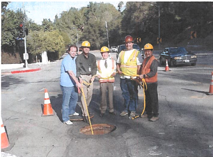
John Gavigan, Vasilij contractor, Mohamad Fakh WCCD, Kendrick Okuda WCCD, Tim Garza-back, Vasilij and Jorge Bustamante Contract Administration.
