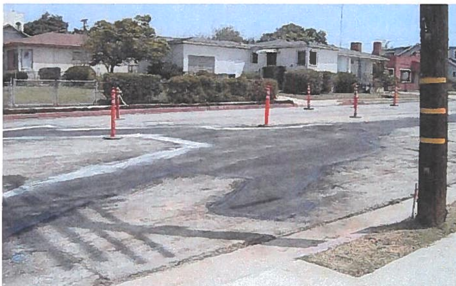
The location of three converging 18 and 21" solid wall HDPE pipe branches is clearly visible in this photo.
