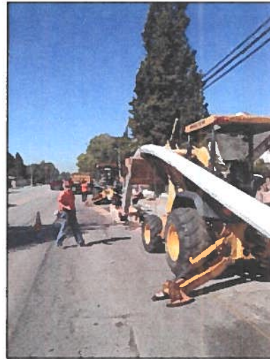
HDPE allowed the city of Covina to install a new pipeline without disruption important community areas like a hospital, baseball field, neighborhoods, and trailer park.
